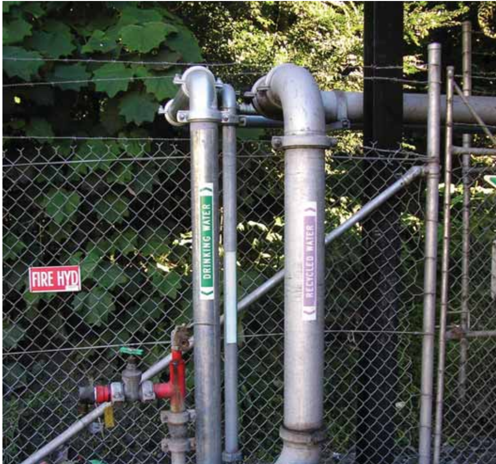
Above: Dendrobium has commissioned a new pipeline to pump recycled water from underground workings to the pit top.
