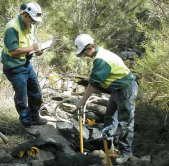
Top: Rehabilitation of Marhnyes Waterhole on the Georges River is now complete.
