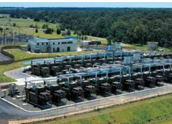
Above: Methane gas from the Appin Mine is converted to electricity at this Energy Developments Limited (EDL) plant.
